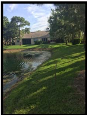
Figure 3: In the background, graded and planted lake bank and in the foreground existing sod area that will be planted with grasses and littorals, so the entire lake bank will be planted with native grasses and littorals.
